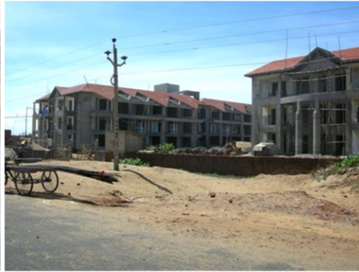
Picture 2: Illegal construction on sand dunes, India
